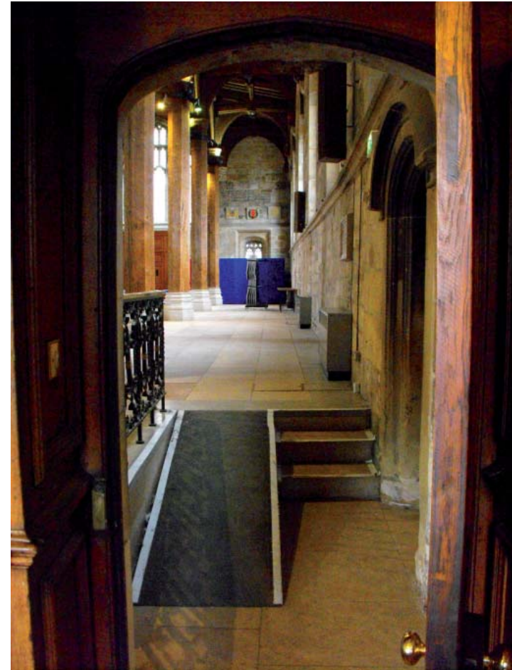
Access improvements to the Guildhall will be a necessary part of any development of the spaces (current non-compliant ramp)
